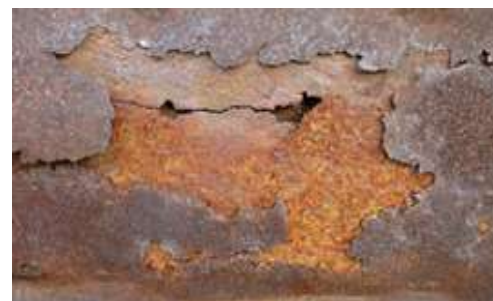
Fig. 4. Corrosion effect in boiler[16]
