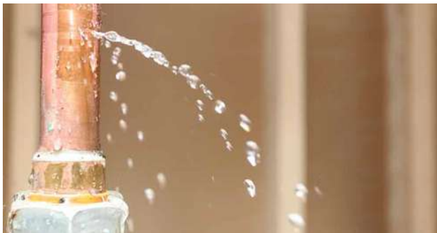
Fig. 3. Leakage of boiler tube[16]
